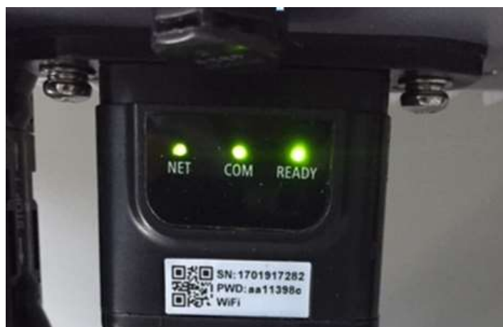
Figure 68 - Final status of LEDs
