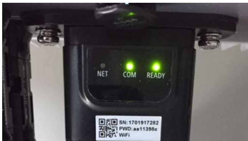
Figure 67 - Initial status of LEDs
